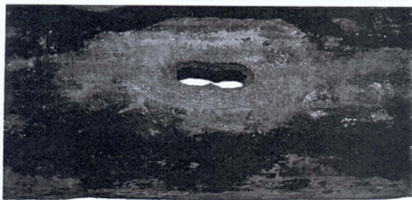
Figure 5. Sample of SPLP destroyed due to external corrosion
