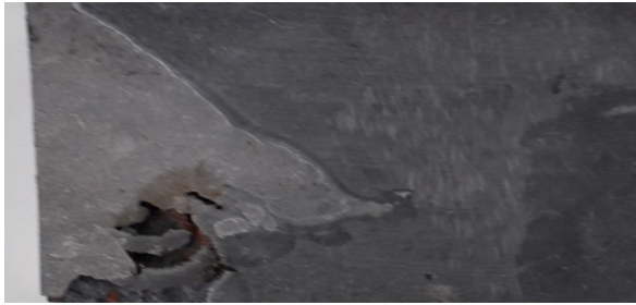
Figure 3. Sample of a welded joint with corrosion damage
