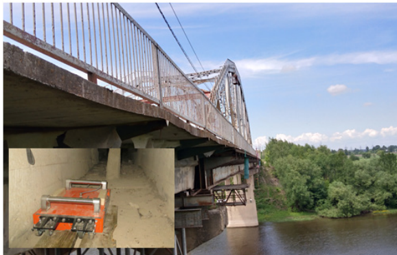
Figure 12. Diagnostics of beams of the «Afanasyevsky» Bridge using the INTROARM flaw detector
