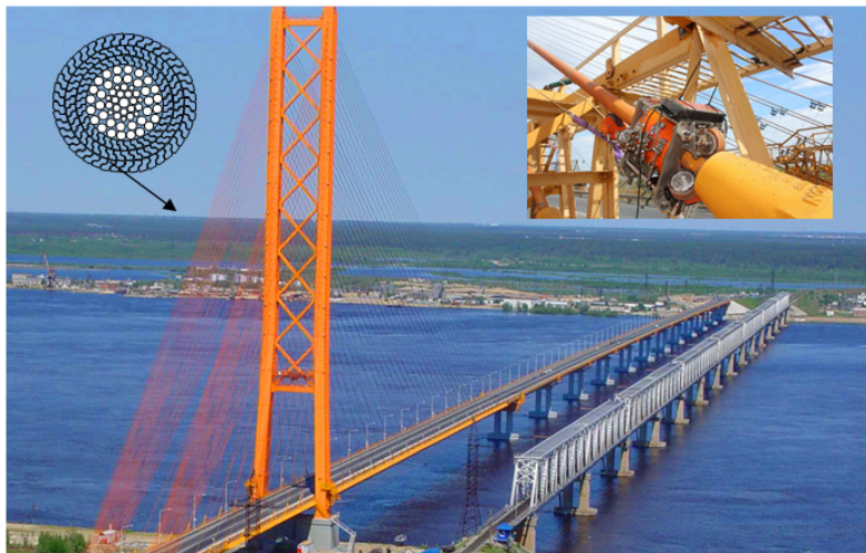
Figure 7. Diagnostics of cable stays of the “Yugorsky” bridge (INTROS flaw detector (MG 60-85))
